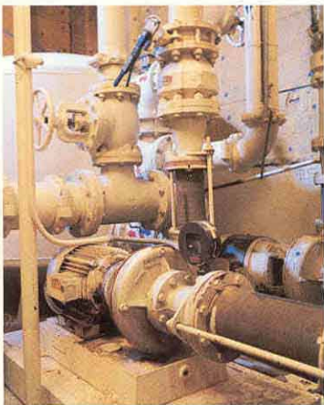
The egret fountain is operated by a 300-gallon-per-minute pump (above) that circulates water from the reflecting pool.
